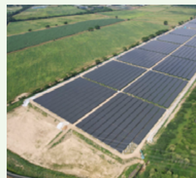
Ground-mounted photovoltaic, Gukeng, Yunlin
