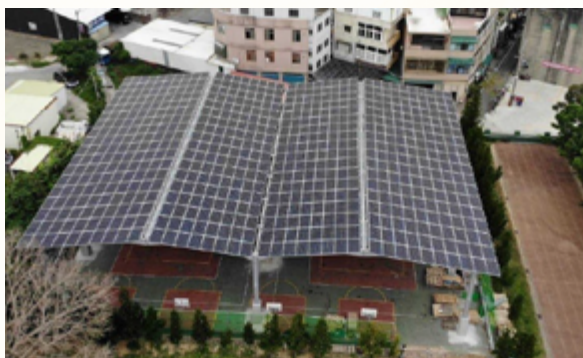
Rooftop solar PV project (Zhuxing Elementary School Basketball Court), Zhunan, Miaoli
