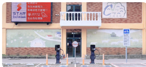
Nantou Cingjing National Guesthouse 17kW*2 Points
